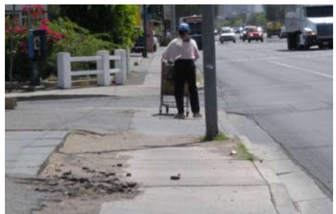
Sidewalk in need of repair.
