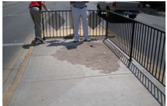
Debris build-up in median area.
