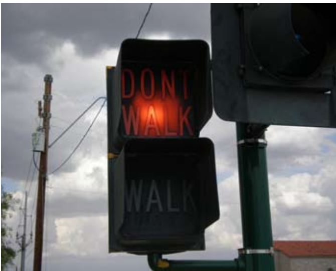
Pedestrian crossing signal requiring replacement.
