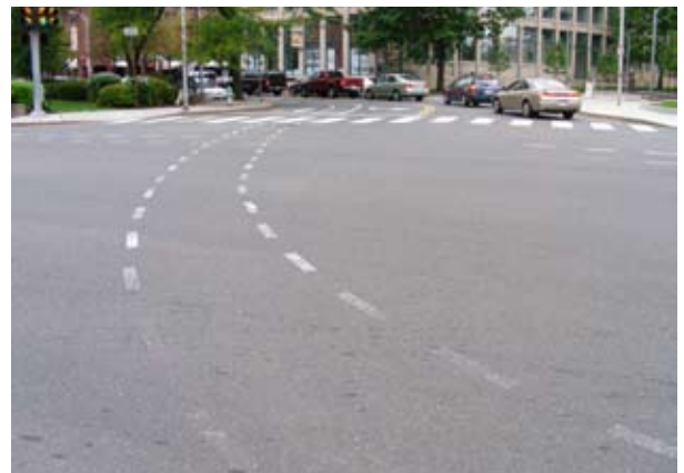
Faded bicycle lane markings.
